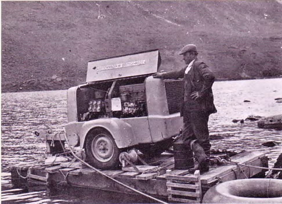
The raft being used as a floating platform for the compressor which supplied the power for the pneumatic drill. The man responsible for keeping the machine going is Mr. S. Vagnarelli ( driver ).
